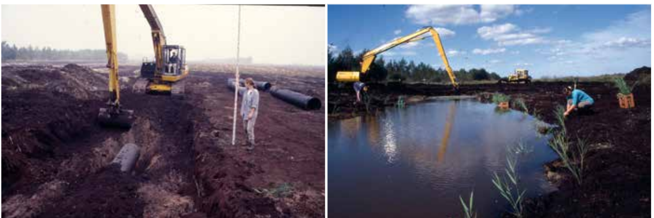
Figures 3 and 4 - Karen Green (Assistant Warden of the RSPB Reserve), on the left with a digger and pipes and, on the right, starting to plant reeds (photo Norman Sills).
