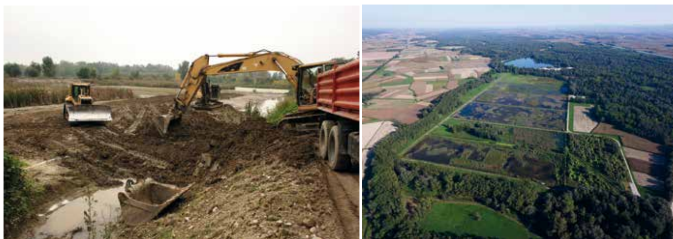
Figures 10 and 11 - New water supply system was built and habitat restoration carried out in the area of ex wastewater basins of the Slovene sugar factory. The area has been declared Ormož Basins Nature Reserve (photo Damijan Denac & Tilen Basle).
