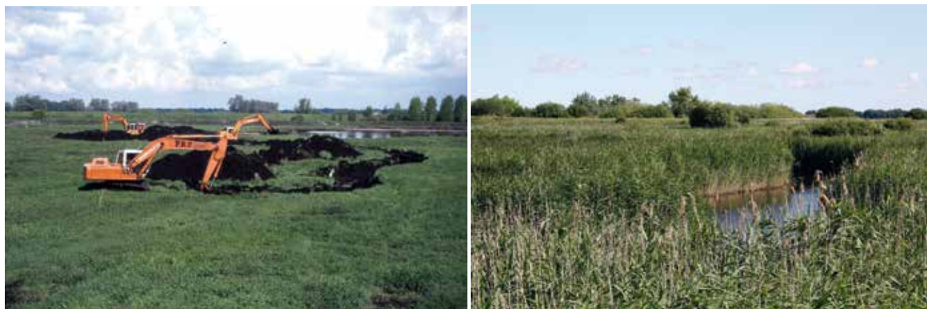
Figures 8 and 9 - On the left: three diggers excavating channels in 2000; on the right: the same place in 2020 (photo Norman Sills).
